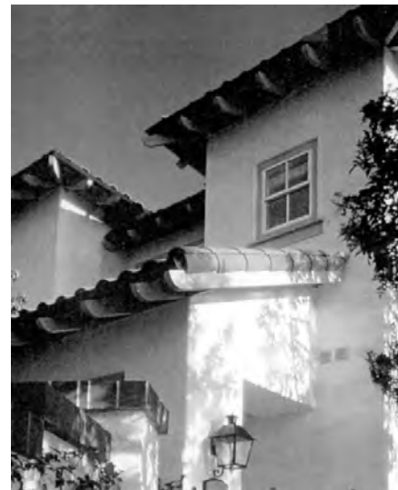
EXPOSED RAFTER TAILS
